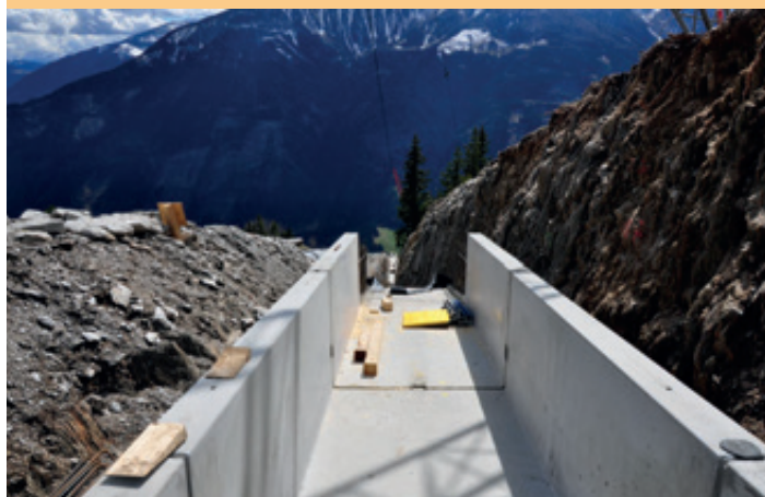
Pump storage power plant, Reißbeck - Austria
